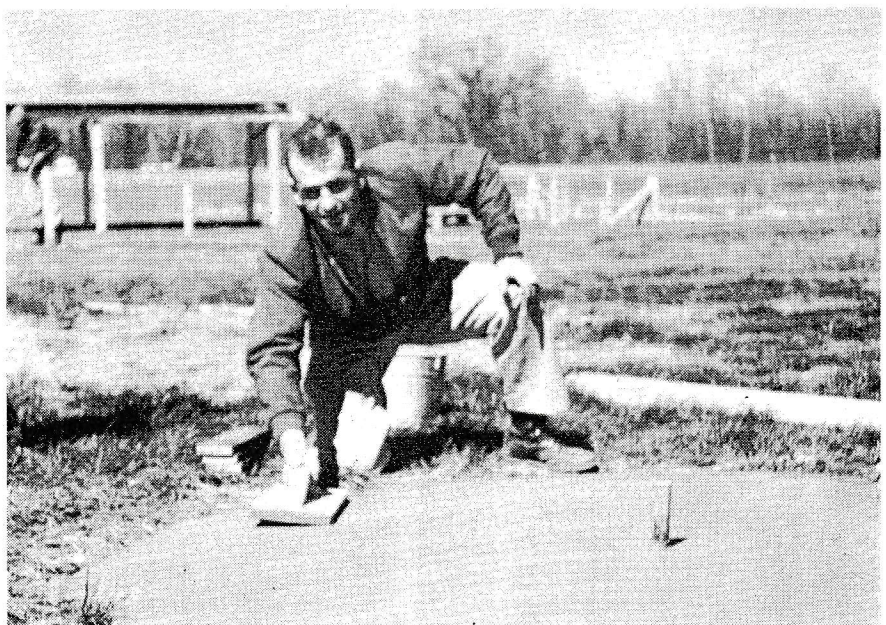
Concrete for center of carrier deck circle is finished off by Charles Eschmann, head of Greater St. Louis Modelers Association. A real working prexy!
